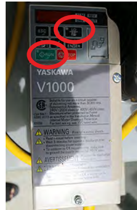
Fan box controls aspirator to remove hulls.
